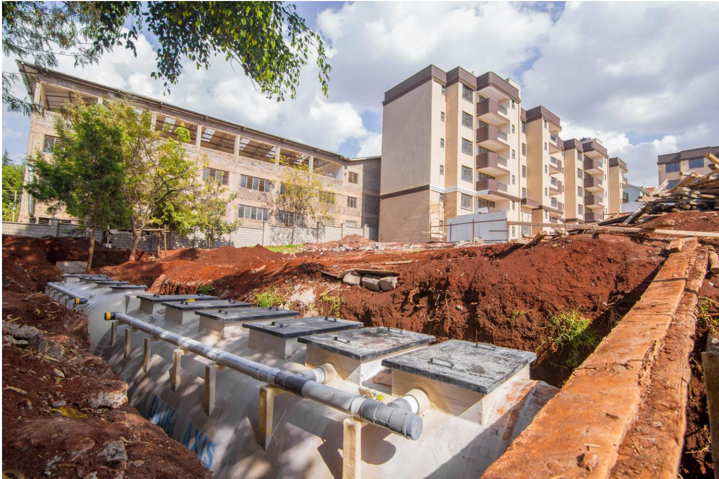
Nairobi Apartment Project 60m 3 /d
