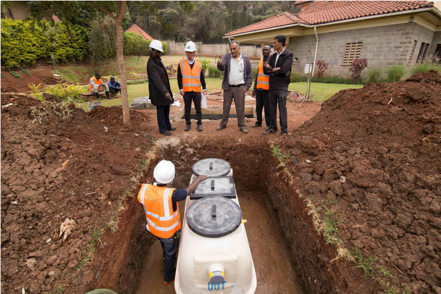
Small scale Johkasou installation_1m3/day
