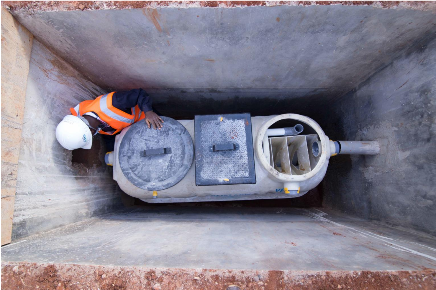
Small scale Johkasou installation_1m3/day
